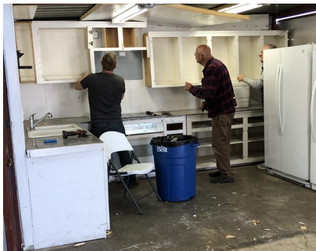
Ian, Tim and Ric, the start of the wrecking crew. It came out quicker than it went in.
